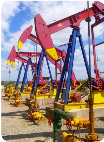
Beam Pumping Unit
