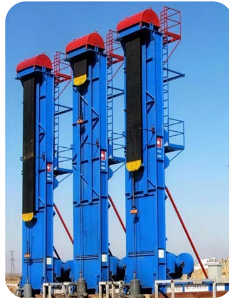
Tower Pumping Unit
